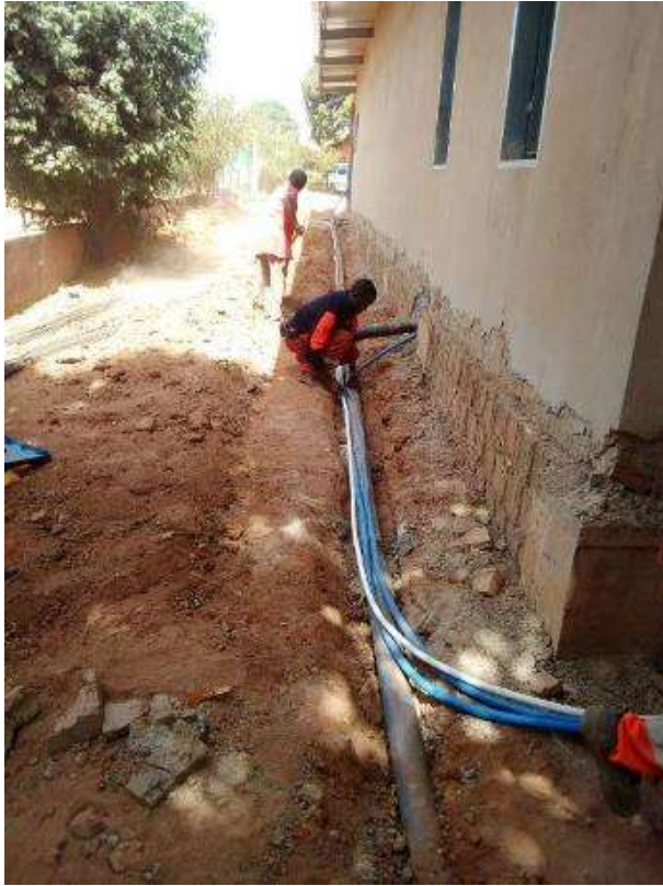
Water pipes and drain sewers laying in the biological pit of the Radiology
