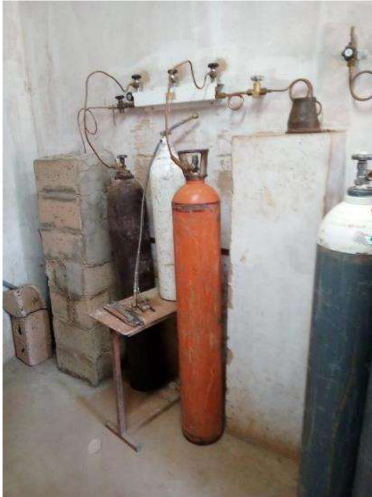
Protective shielding with reinforced concrete of the 2 oxygen loading lines in cylinders for technical staff protection
