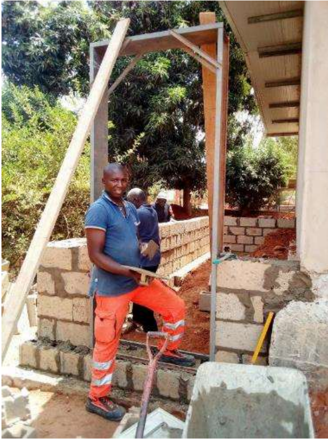
Construction of the cabin containing the general electrical panel for radiology pavilion
